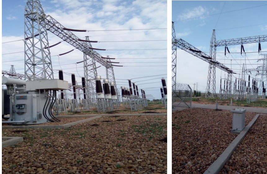
Figure 3: Renk Substation. Photo by Jok Gai, September 2017
